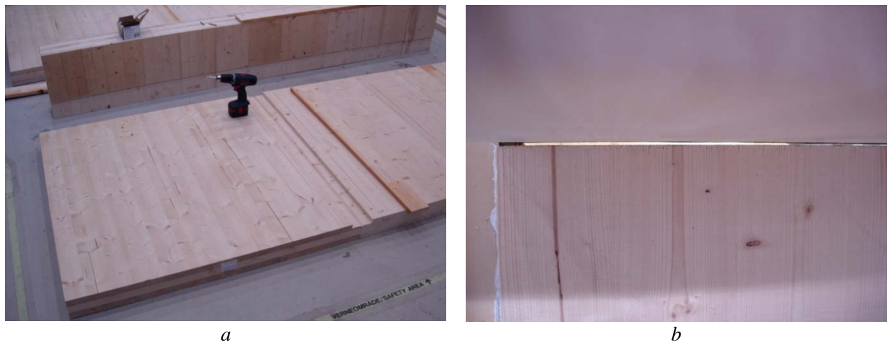
FIG 5. Mounting of the cross laminated timber test section. The joint between the wall elements are covered with a spruce board fastened with screws (a). Typical gap between the wall and floor element caused by rough and uneven surfaces (b).
