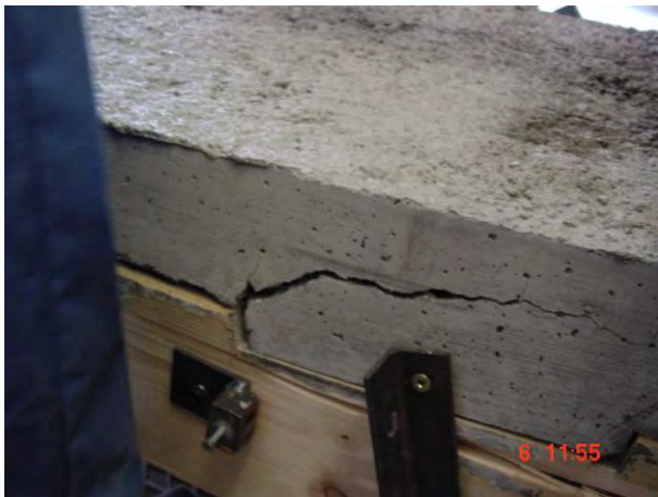
Cracking of concrete
